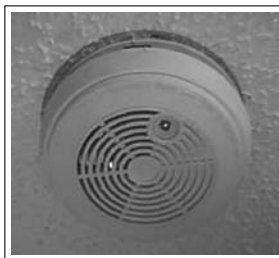
Figure 3. Residential ceiling-mounted smoke detector.
